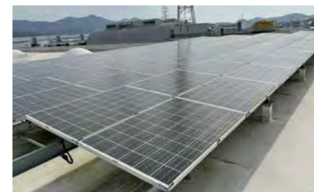
Topura Hadano Plant (20kW, Start from FY2012)
