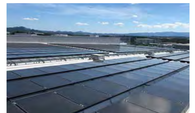
Tokuhatu Sanda Plant (120kW, Start from FY2016)
